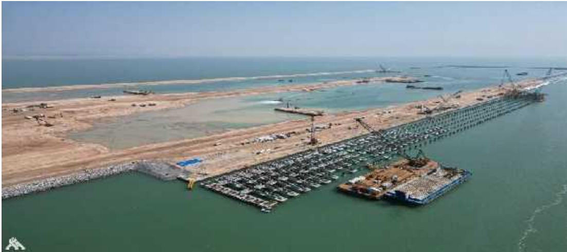
Figure 3. The five main berths have been completed in the port of Faw Source: Iraqi ministry of transport 2023
