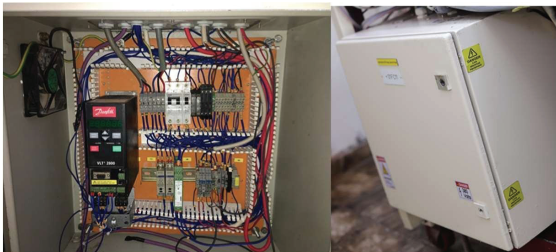
Figure 6. The third control panel contents
