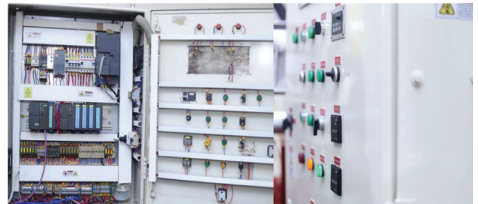
Figure 5. The second control panel contents
