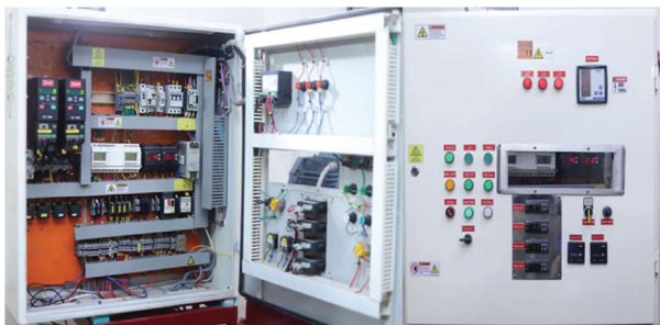
Figure 4. The first control panel contents
