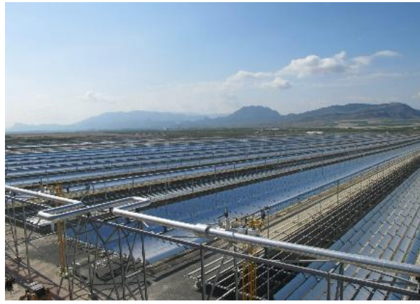
Fresnel Flat Mirror Technology, Puerto Errado in Spain, 30 MW with 0.5 hours Storage
