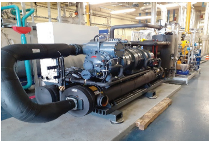
Fig. 7. Rear view picture of the heat pump
