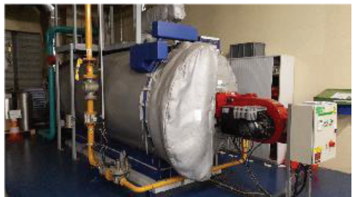
Fig. 3. Hot water boiler
