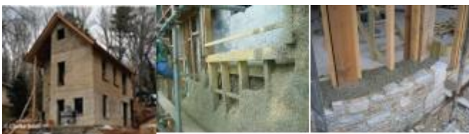
Fig.2. Shows that hempcrete can be cast manually around a timber frame using a shuttering system,
