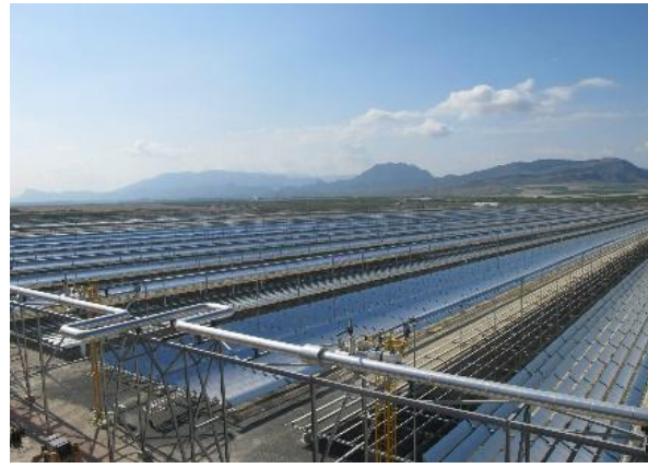
Fresnel Flat Mirror Technology, Puerto Errado in Spain, 30 MW with 0.5 hours Storage
